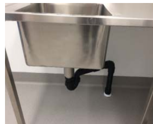
Sealed floor penetration (using flange sealed to floor)
