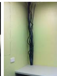
Exposed electrical cables
