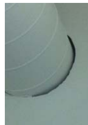
Unsealed ceiling penetration
