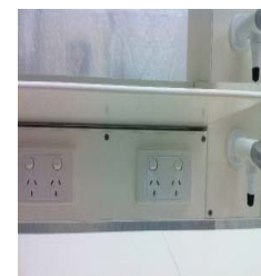
Electrical wiring enclosed within service duct
