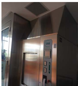
Autoclave enclosed to ceiling
