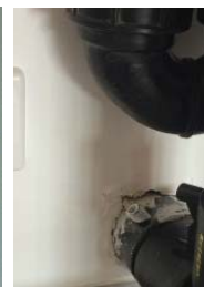
Unsealed wall penetration
