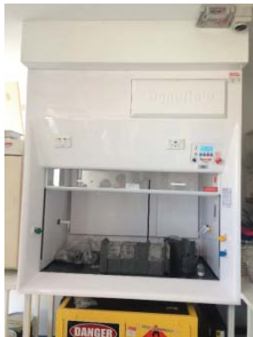
Fume cupboards bulkhead to ceiling
